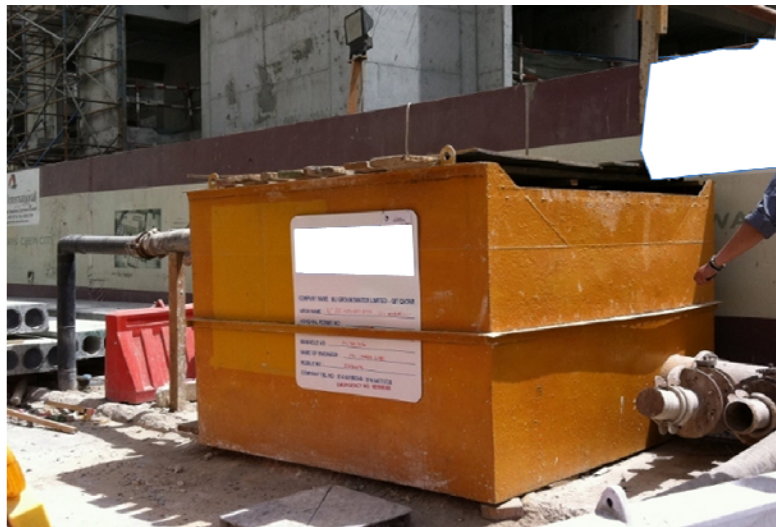
Figure 3.6 Typical Settlement Tank Used in Qatar
